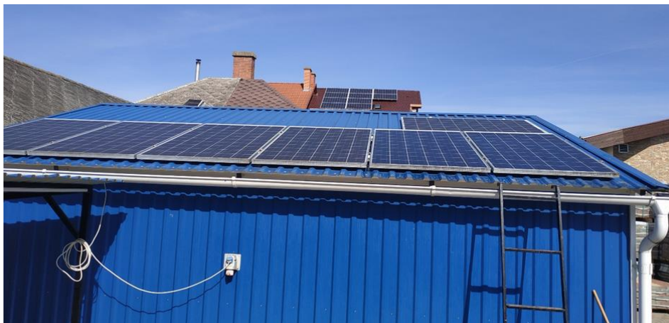
5. Figure: Measured solar panels on the roof of a garage.
